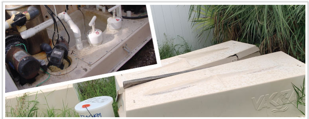
Photos courtesy of Commercial Energy Specialists (CES)—Before photos (not Regatta)
